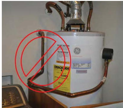
BAD: T&P discharge should flow with gravity and be observable
