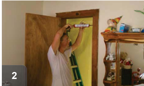
Foam, caulk, and seal leaks between halves of double wide manufactured homes
