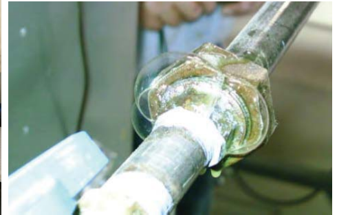
If bubbles develop, leak is present. Notify occupant
