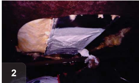
2 Mobile home duct systems (plenum, trunk terminations) should be sealed from below prior to patching the belly.
