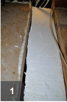
Chase has been capped but needs to be sealed
