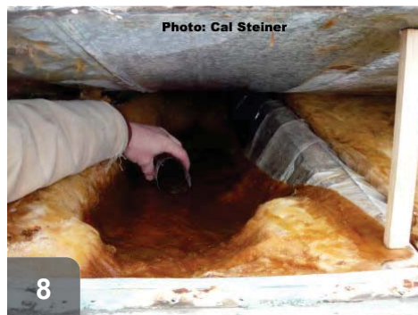
8 Investigate all water stains and sources of moisture. Repair before insulating the attic
