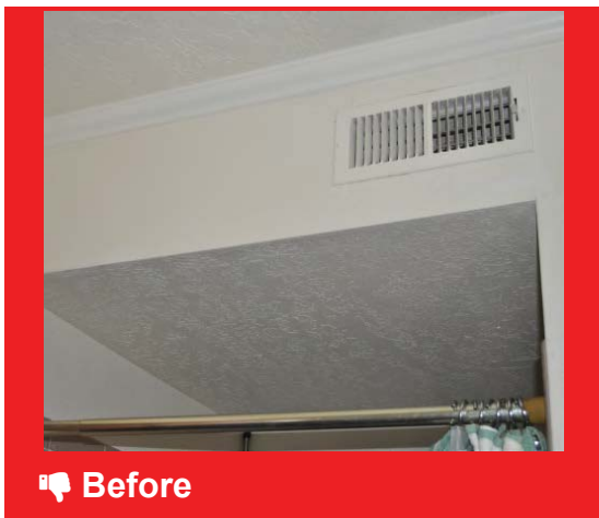
Standard soffits are often open to the attic and uninsulated
