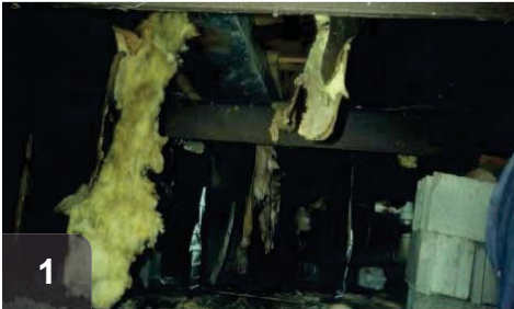
1 Belly damage: rodent barrier and insulation are damaged, revealing a main supply duct known as a trunk.
