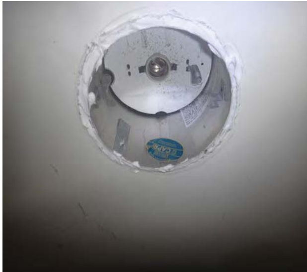
IC rated recessed fixture air sealed from the interior of the home.
