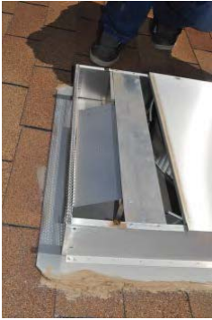
Backdraft damper on roof mounted exhaust fan
