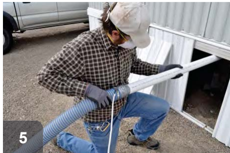
Blow in insulation with peace of mind that workers will not be electrocuted
