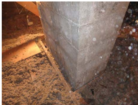
Air leak around masonry chimney, needs to be air sealed.
