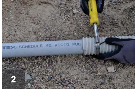
2 Attach grounding wire to fill tubes to minimize shock risk
