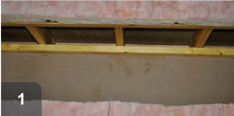
Soffits open to the attic need to be sealed to maintain air barrier
