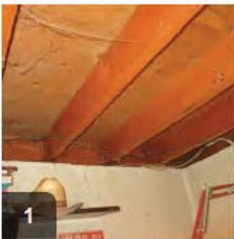
1 Rim joists in a conditioned basement lack pressure and thermal boundaries.
