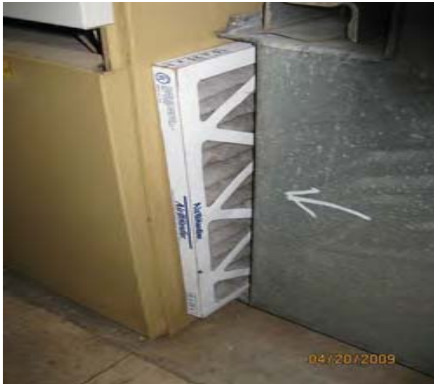
Furnace filter slots located in the return plenum are often leaky, creating depressurization in the zone.
