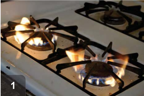
Yellow, uncontrolled flames indicate the need for a clean and tune
