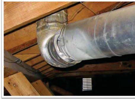
Inspect ventilation systems for damage
