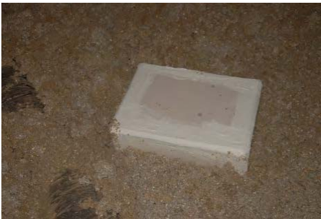
Non-IC (insulation contact) can lights should be covered with a dam and have no insulation on top
