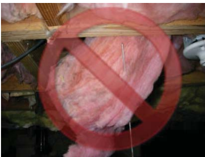
Wire batt support rods (known as tiger teeth) are prohibited because they compress insulation, rust, and fall out.
