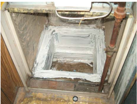
Plenum to duct trunk connection coated with mastic sealant
