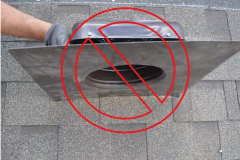
BAD: Termination fittings without collars should be avoided
