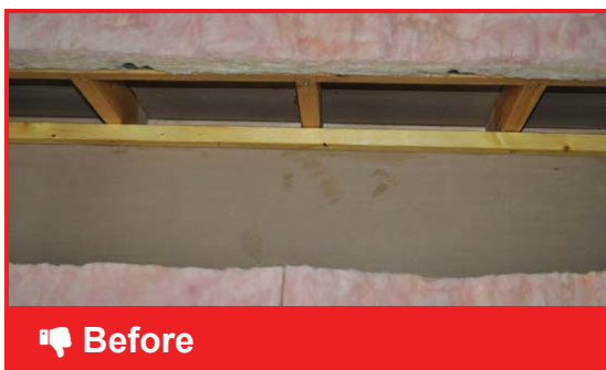
Unsealed drop soffits over tubs and closets can be a point of leakage
