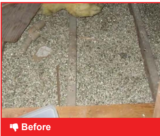
Material identified as vermiculite may contain asbestos
