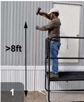
Copper grounding rod should be at least 8' long
