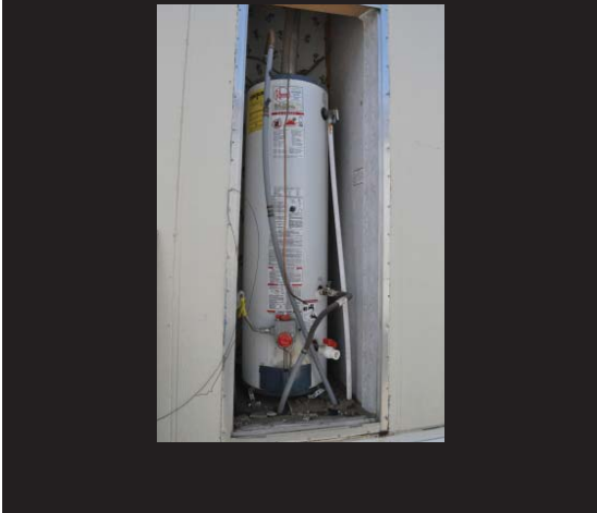
Standard water heaters have built-in insulation ranging from R-7 to R-20.
