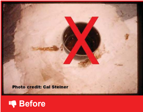
Roof leak, missing cap on vent
