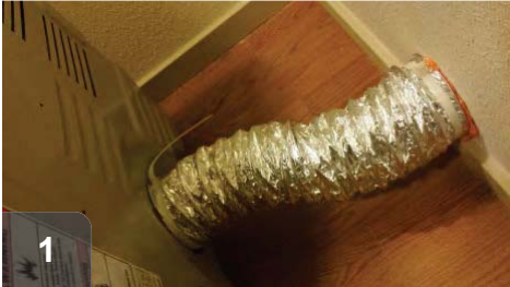
1 Dryer vent transition piece: panduit straps, metal collar at wall, foam air sealing
