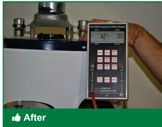
Test combustion appliances for spillage to confirm they comply with combustion safety standards.
