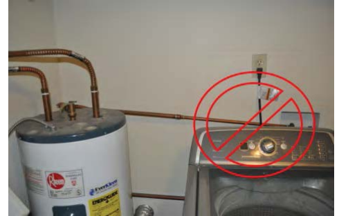
BAD: T&P discharge should not be piped into drainage system
