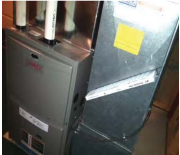
Furnace filter slots located in the return plenum are often leaky, creating depressurization in the zone.
