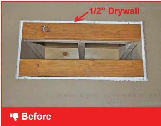
Unsealed standard chases covered with drywall can be leakage points
