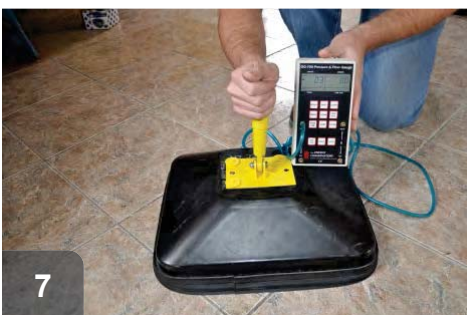
7 All duct sealing and repair will be confirmed with pressure diagnostics.
