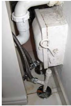
Electrical wiring should not be located near a water source
