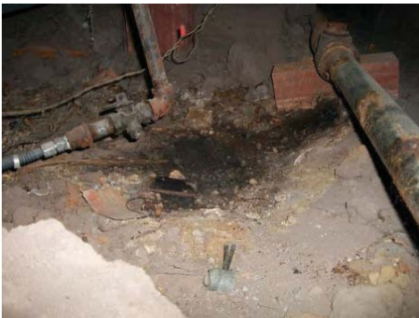
Any leaks found should be reported to occupant and work stopped
