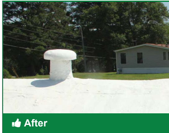
Properly connected and sealed roof vent
