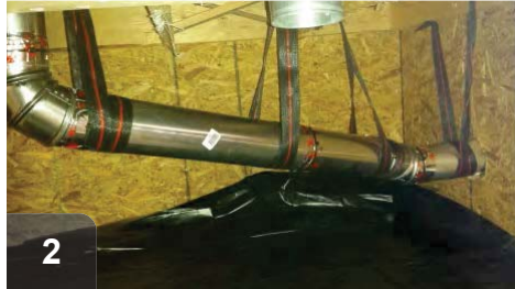
2 Uninsulated dryer venting in unconditioned space
