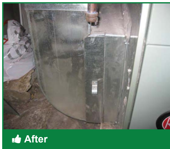
Filter slots should be covered
