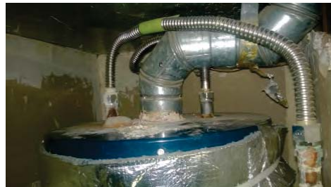
Inspect for missing draft diverter
