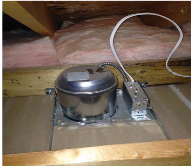
IC rated recessed fixtures can also be sealed from the attic when accessible.
