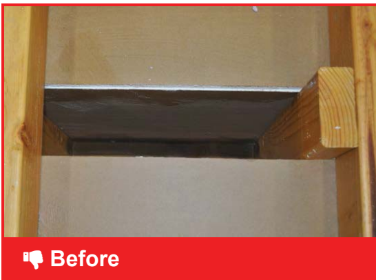
Wall cavities are open to attic
