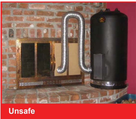
Unsafe solid fuel burning appliances should be replaced
