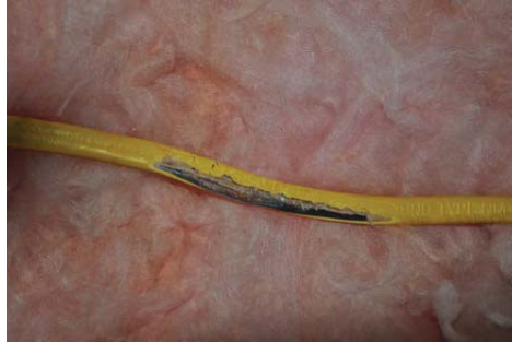
Check for frayed or worn electrical wires
