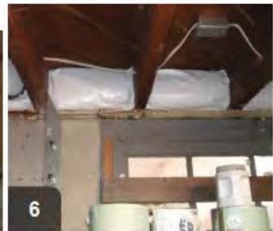
6 Fiberglass needs vapor retarder facing. FSK batting or metal building insulation (MBI) are acceptable.
