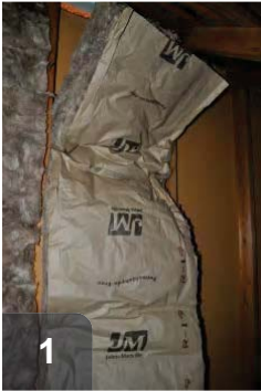
1 Where existing insulation is improperly installed, fix it
