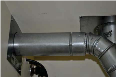
Inspect ventilation systems for inadequate slope
