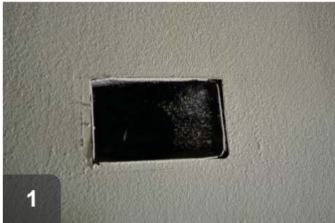
Remove grill to expose duct boot and gaps
