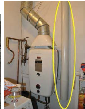
Ensure there is adequate make-up air -- combustion air inlet in closet
