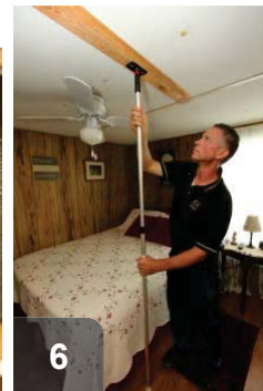
6 Use temporary supports to avoid ceiling collapse during insulation install
