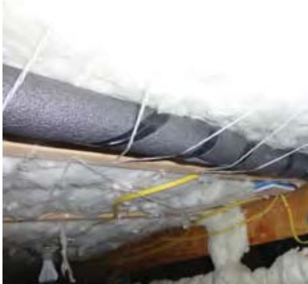
Water supply lines insulated with R-3 foam pipe wrap
