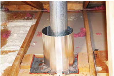
Damming is held in place with mechanical fasteners and maintains 3" clearance from flue.
