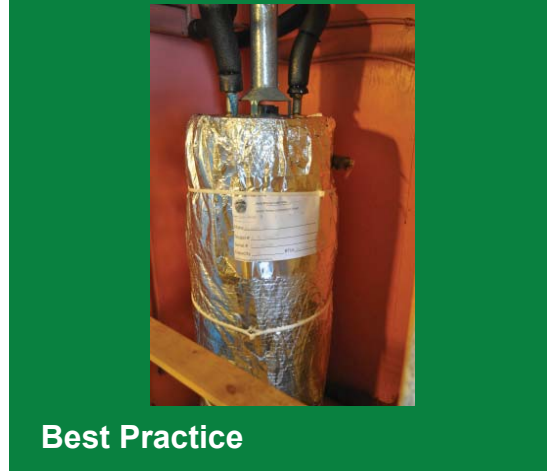
Storage-type water heaters should be wrapped to bring total value to R-24
