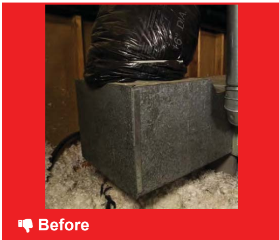
Duct to plenum not sealed
