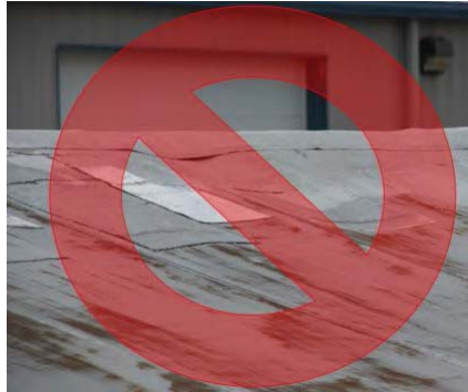
Dishing and pooling issues must be addressed.
