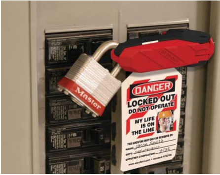
For electric furnaces, follow lockout/tag-out procedures to break circuits that supply furnace with electricity.
