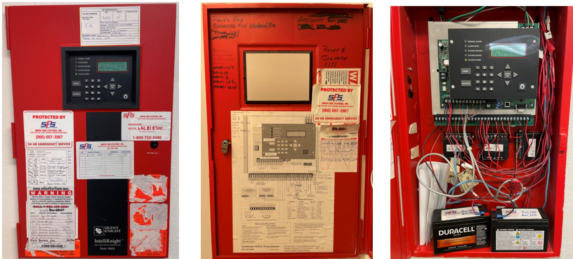
Main Fire Alarm Control
