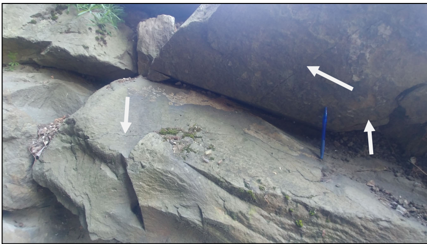
Figure 2. Typical cracks in existing rockery boulders.
