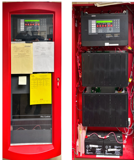
Main Fire Alarm Control
