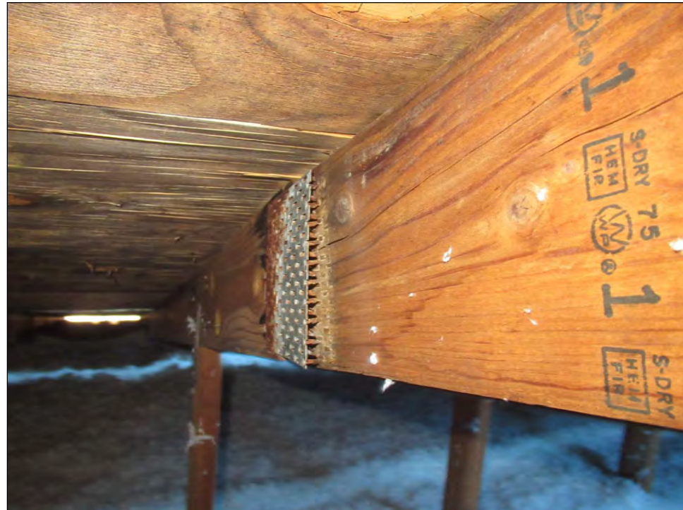
TRUSS SPLICE PLATE DAMAGE
