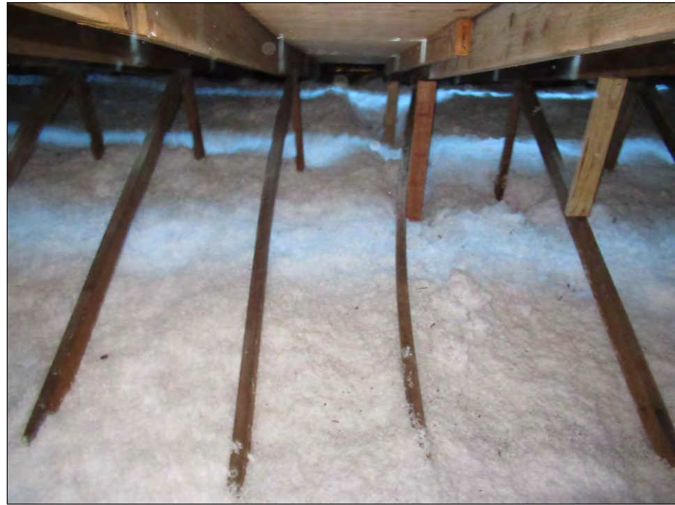
DAMAGED ROOF TRUSSES
