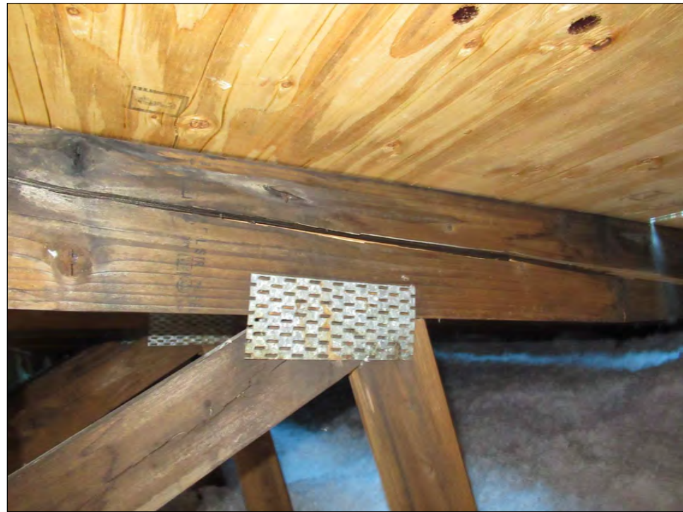
TRUSS TOP CHORD FRACTURED
