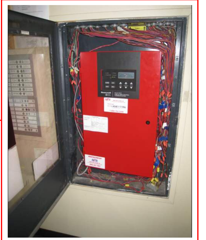
FIRE ALARM CONTROL PANEL
