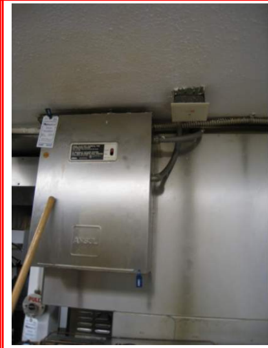
KITCHEN HOOD ANSUL SUPPRESSION SYSTEM
