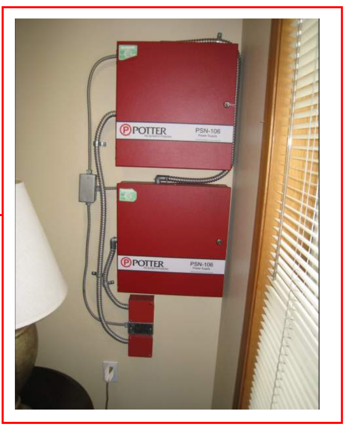
FIRE ALARM POWER SUPPLIES
