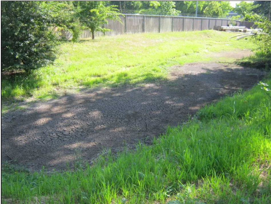
9. Artificial stormwater retention pond
