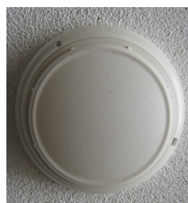
Common Area Smoke Detector
